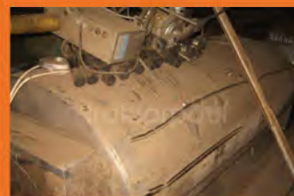
1616842 Mullerup Cooling tank
